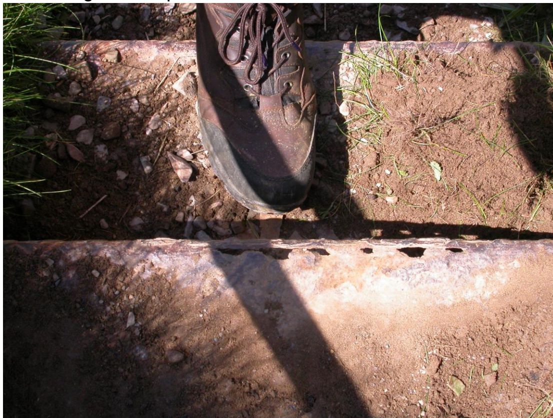
Steel step tread showing severe corrosion and closed chequer plate construction
